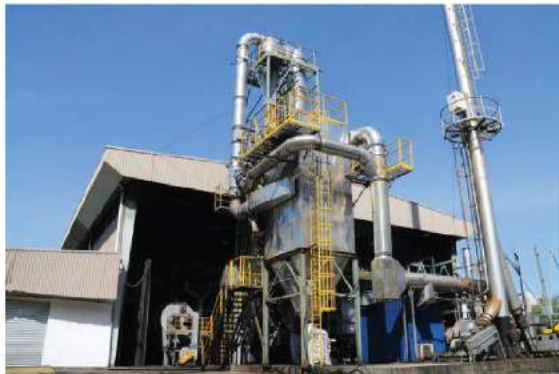
AFES operates Pulau Pangkor Incinerator
